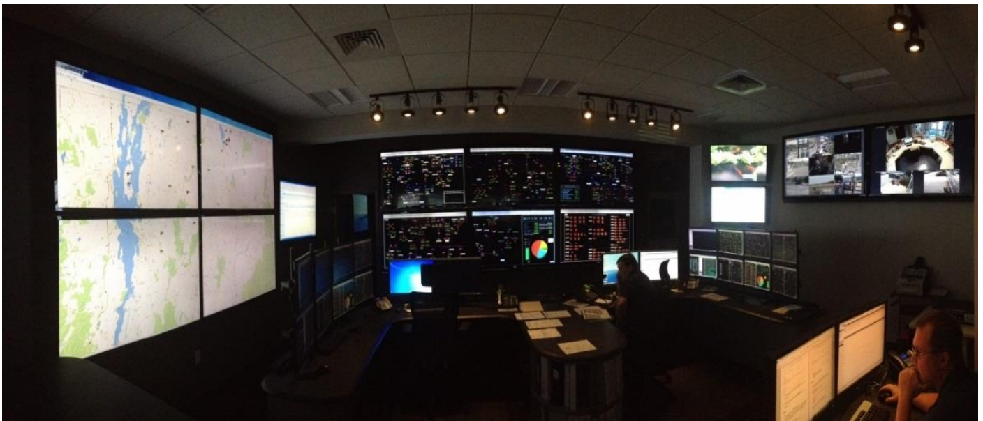
Figure 4.7.5.A VEC control room
