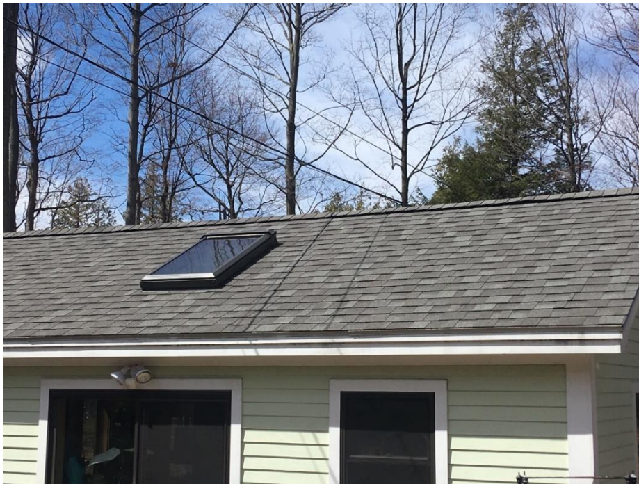
Figure 4.2.1.B NESC violation above addition in Grand Isle, Vermont
