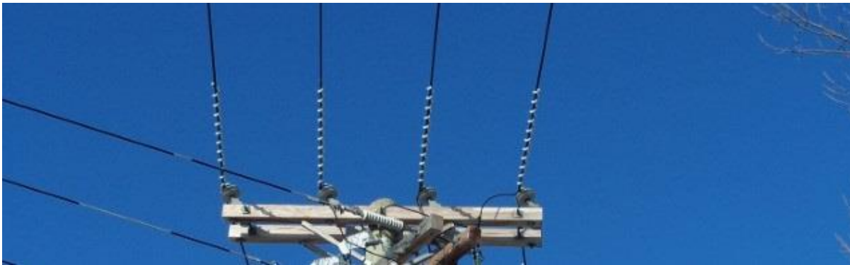
Figure 4.5.12. Covered conductor (“tree wire”)
