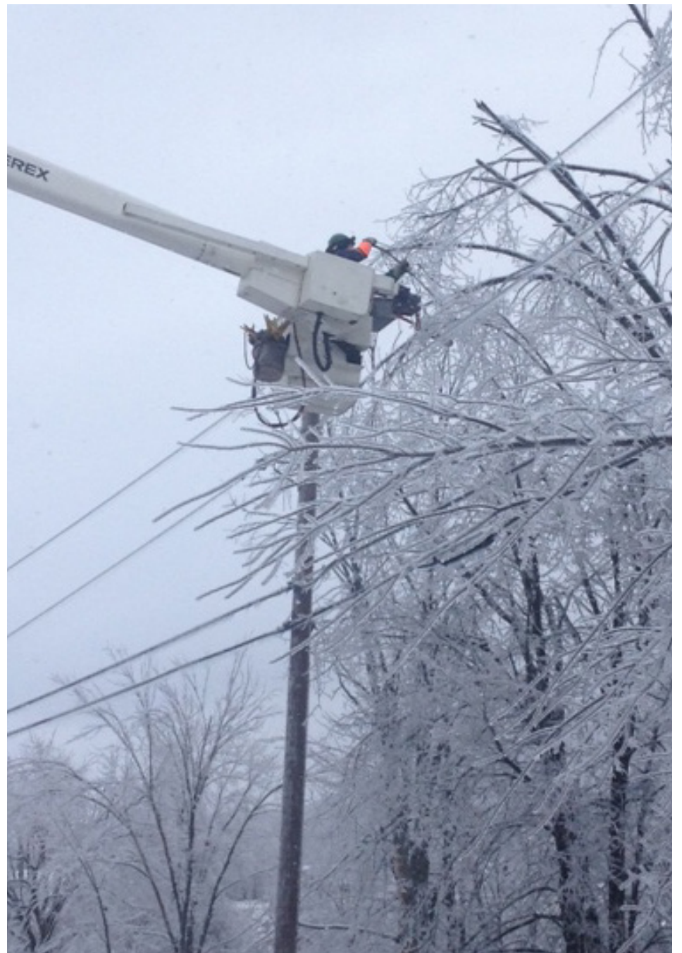
Lineworker repairing a line during the December 2013 ice storm, which caused thousands of outages.
