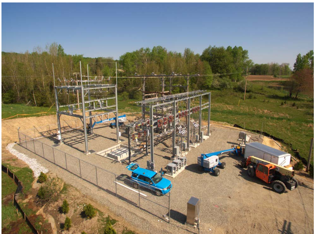
VEC's East Berkshire Substation, pictured here under construction in 2016, is one of 35 substations located across VEC territory.
