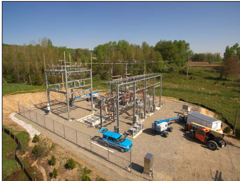
Substations, like the East Berkshire Substation above, are key to keeping the power flowing to our members.
