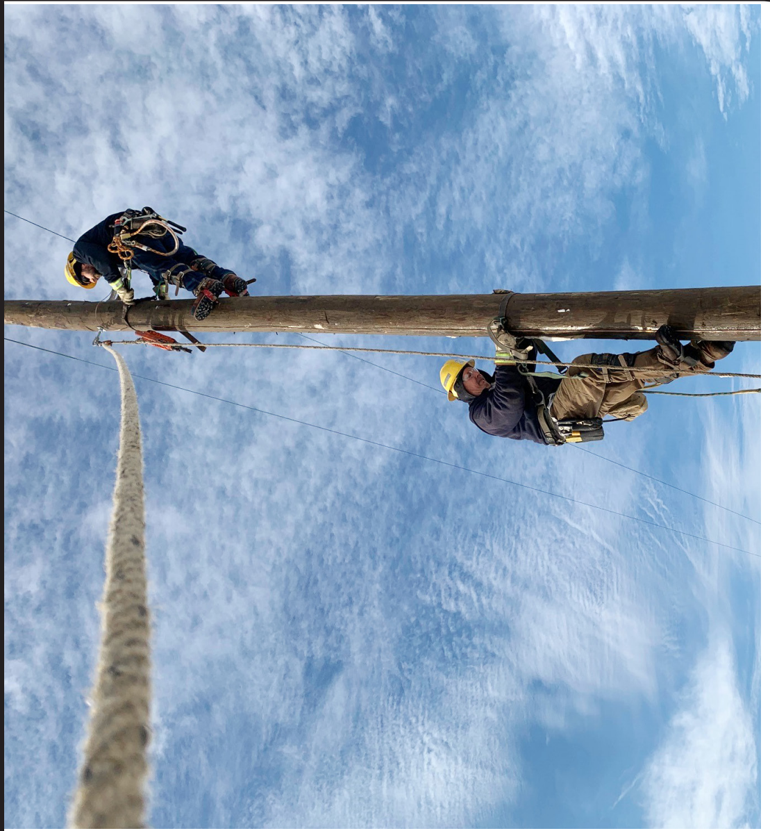
Fred Jewett (left, toward bottom of pole) and Ryan Nieckarz replace a broken pole in Berkshire after winter storm Elliott.
